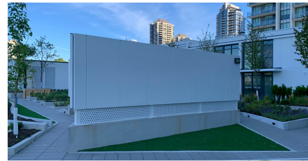
Ld-5 Reference image for VRF Screen - Size to be determined L-1.1/1.4 NTS
