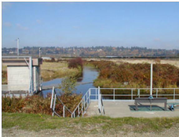
Mud Bay Pump Station
