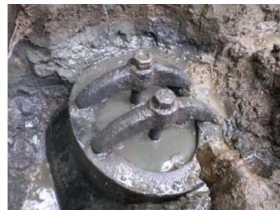
Siphon Blow Down
