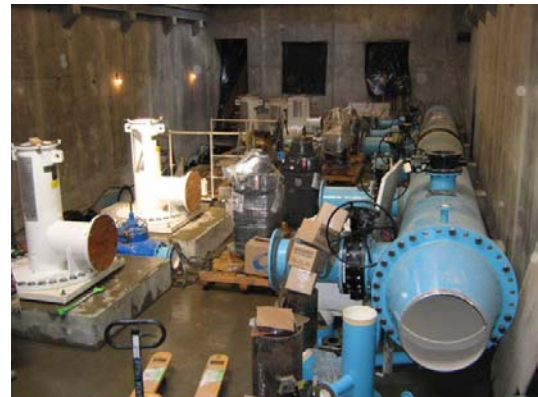
Clayton Water Pump Station
