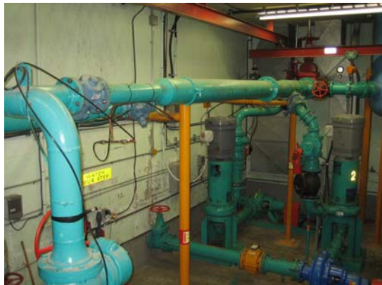
Semiahmoo Pump Station
