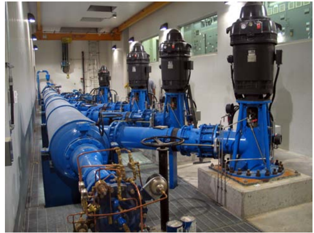
Inside of the Grandview Heights Water Pump Station
