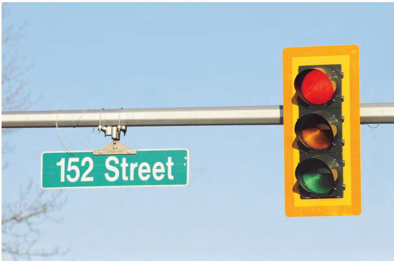
152 Street streetlight for Roads & Traffic Safety
