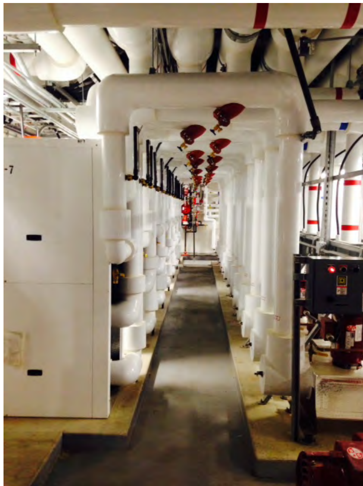
Surrey City Energy for New City Hall
