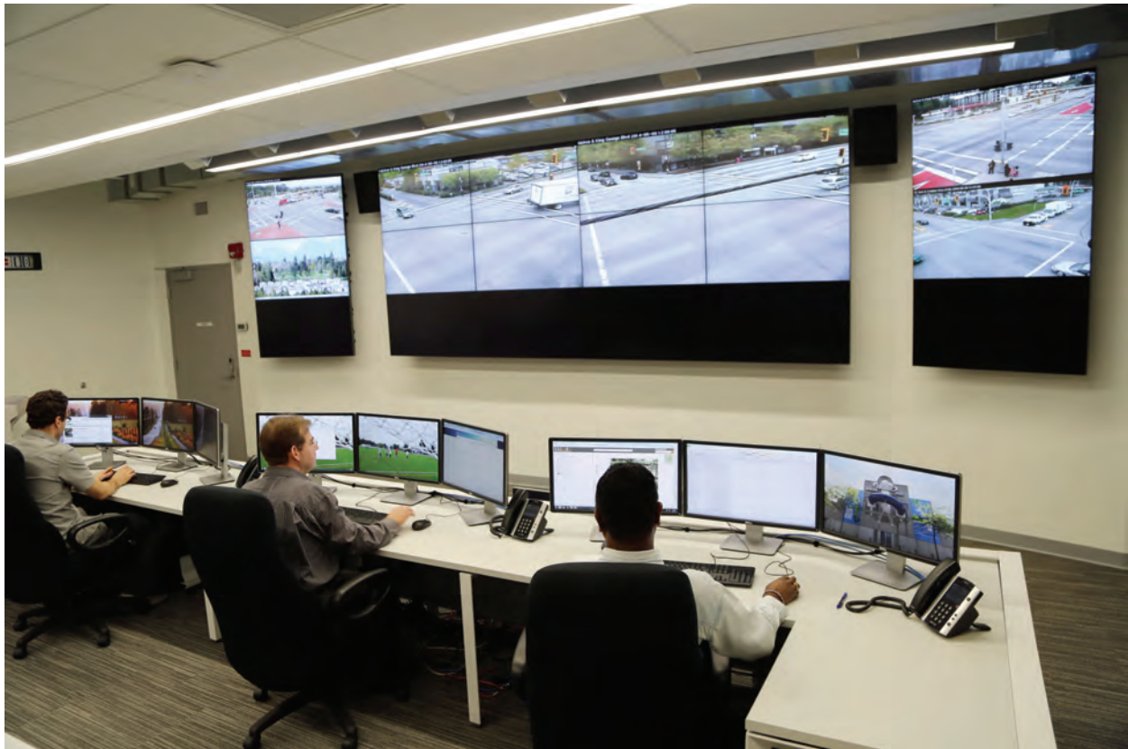
Traffic Management Centre
