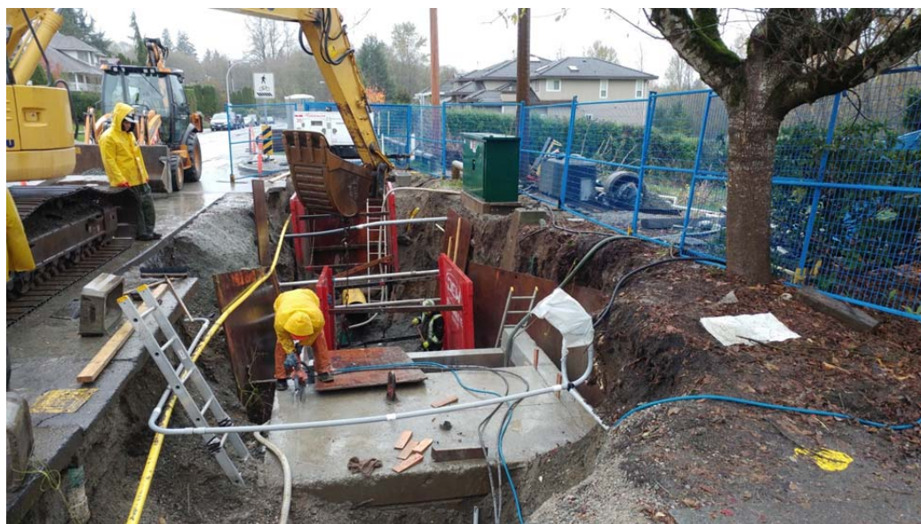
95 Avenue and 164 Street PRV
