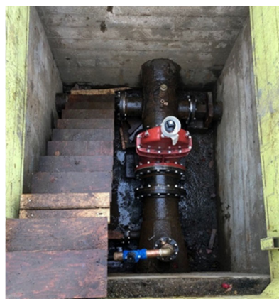
Water Valve Chamber
